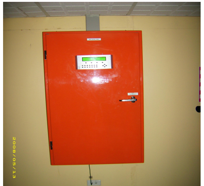
SWITCH BOARD INSTALLED
