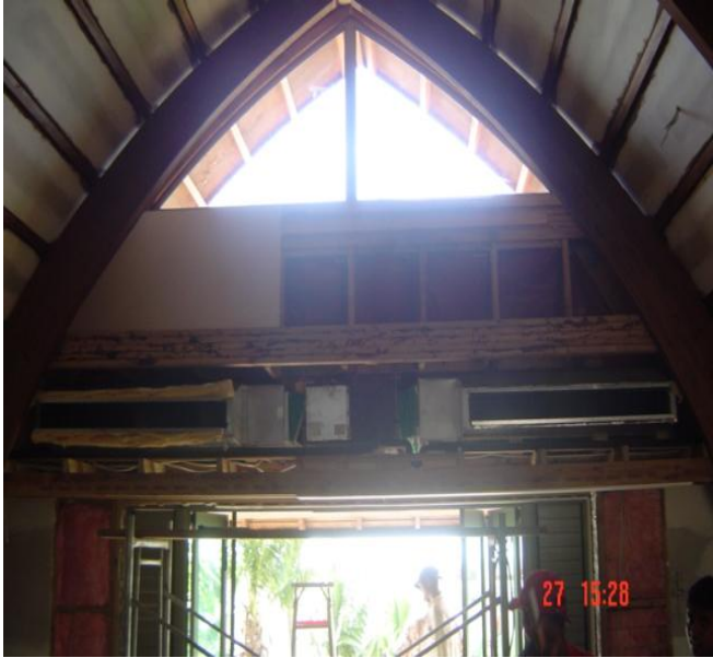
VRV IIS INSTALLED
