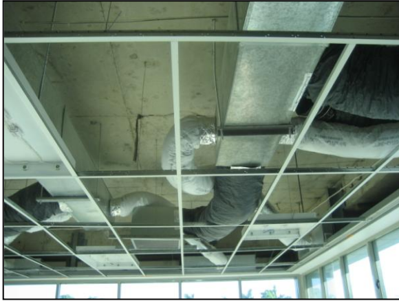
Supply duct and flexible
